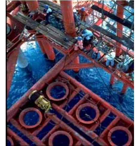
Offshore rig workers lower a large drilling template into the ocean. It will guide the platform's drilling by providing an anchor to the ocean floor.
