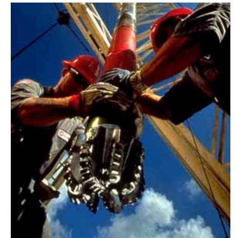
Workers lower a new rotary bit into the wellbore. Notice the sharp teeth that will break up rock formations.
